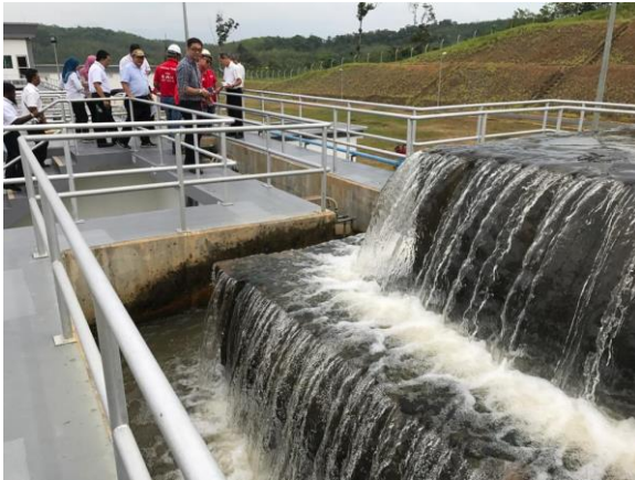
Aerator at Kuala Kangsar Treatment Plant
