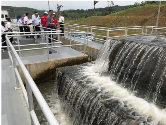
Aerator at Kuala Kangsar Treatment Plant
