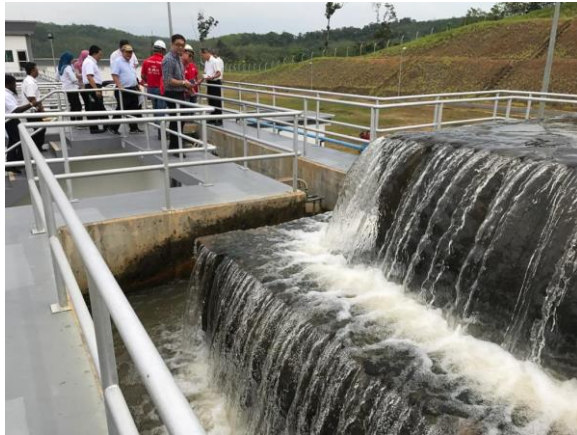
Aerator at Kuala Kangsar Treatment Plant
