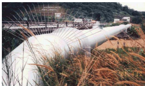
Proposed Joint Water Supply Main at Mukim Tanjung Dua Belas Daerah Kuala Langat, selangor Darul Ehsan (Stage 1) for :-
